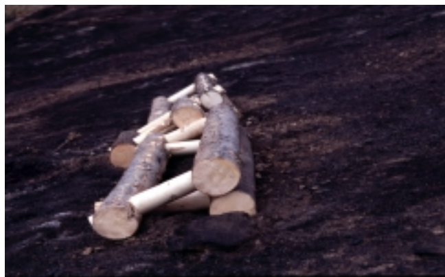
Figure 7.—FlowCheck™ hillslope erosion control materials are constructed from smallwood as an alternative to cross-felled trees and straw wattles.
